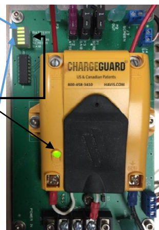
New Style Circuit Board
